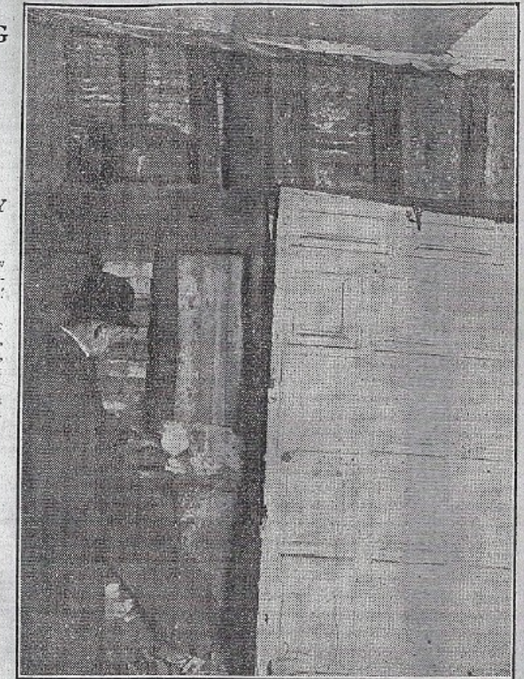
Picture gives some idea of the composition of the walls of an old house now being demolished in Butcher Row. Walls being brought to light through the removal of panelling show that the spaces between the beams were filled in with clay and straw.
